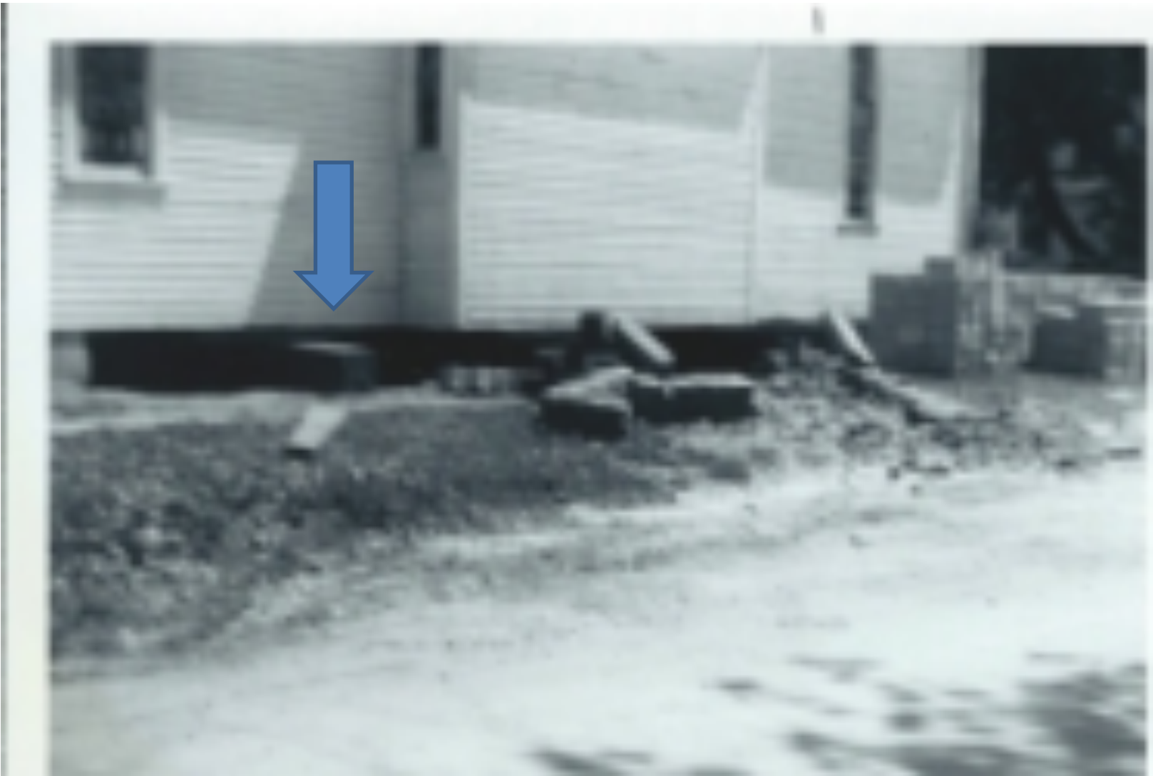
The church was jacked up slightly to accommodate the supporting walls of the basement. The arrow shows another large supporting timber while the basement was being dug.
