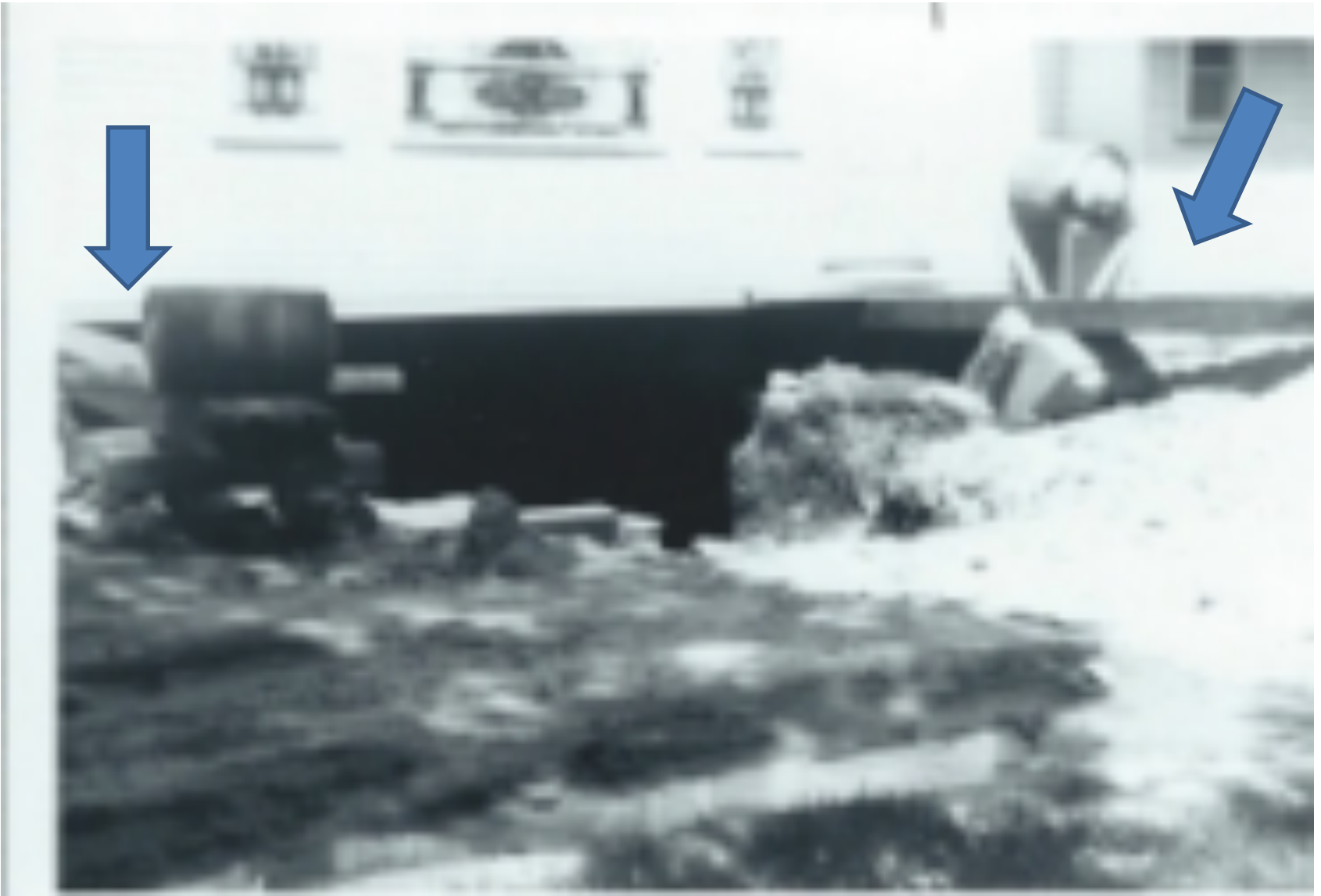
This was no easy feat as you can see the size of the big timbers put under the church.
