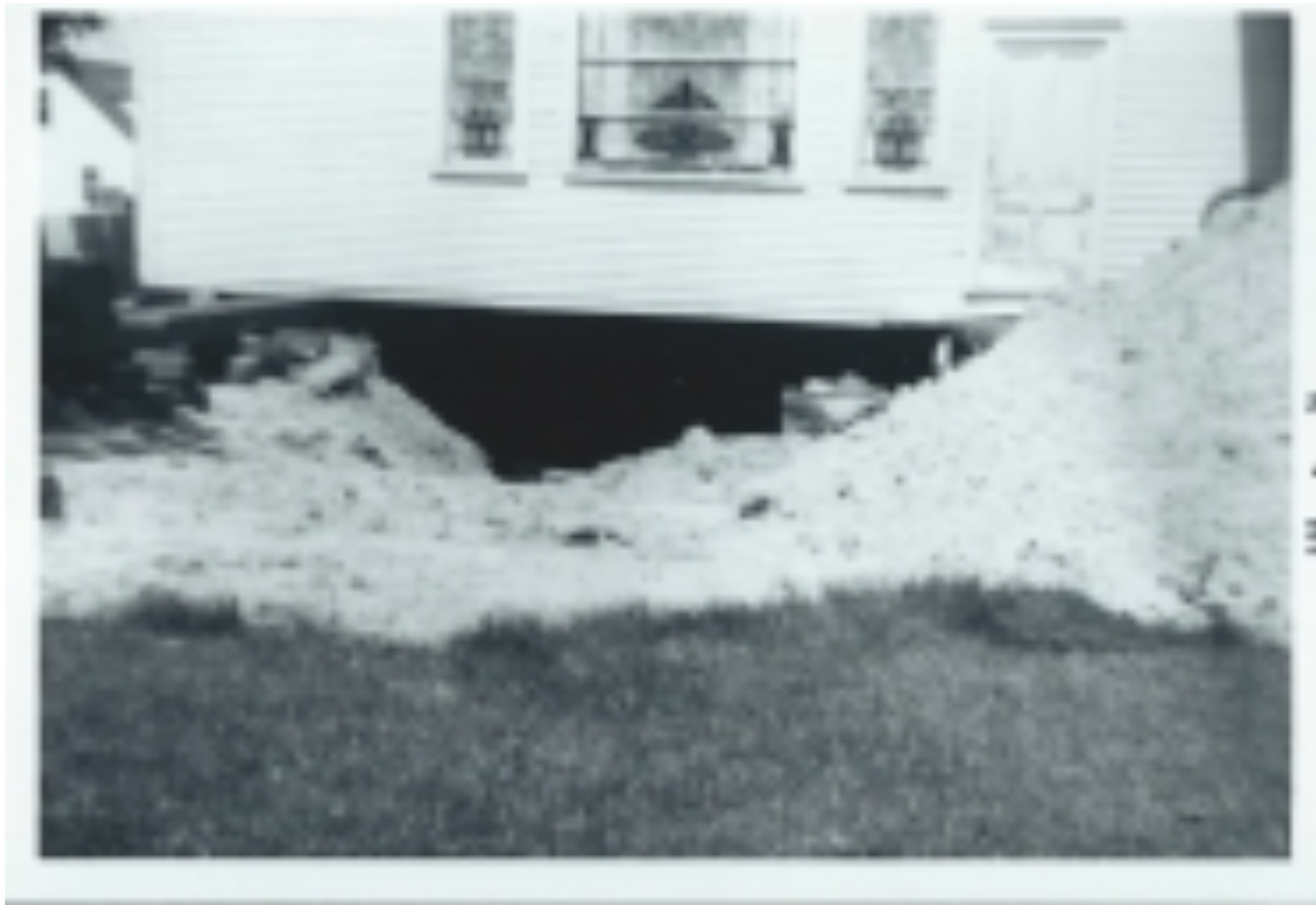
In the spring of 1955, it was decided to dig a basement for the church.
